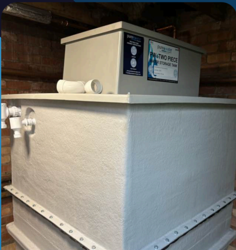
New water storage tank
